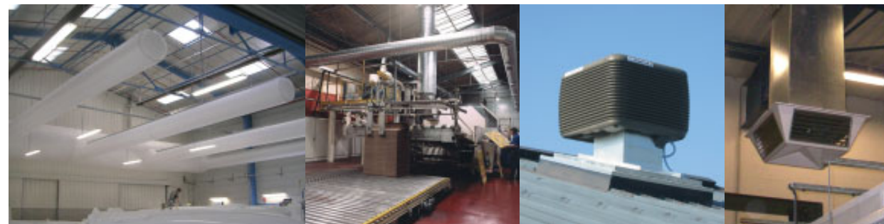
Diffusion of cooled air via textile ducts
