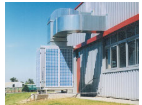
Cooling in a workshop by Econoclim® C
